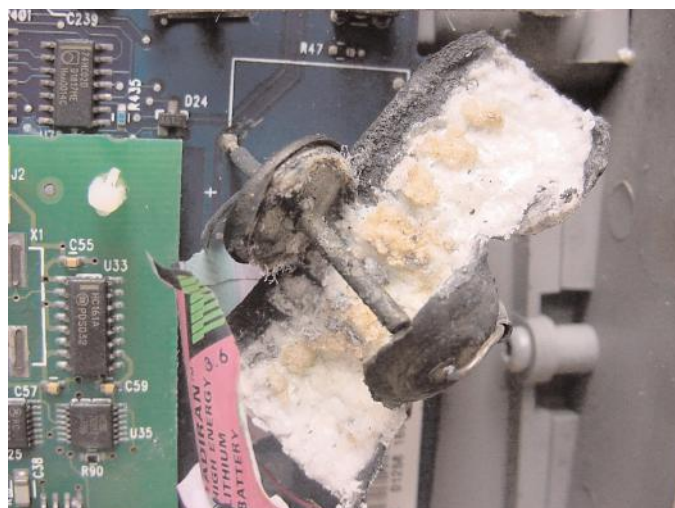
Incorrect Batteries can corrode and cause more damage.
