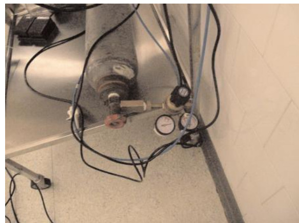
Incorrect storage of a cylinder
